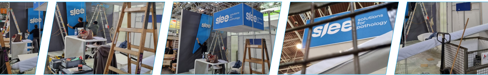
Sunday morning. Still building up. On Monday morning, the booth was ready, nice and shiny!
